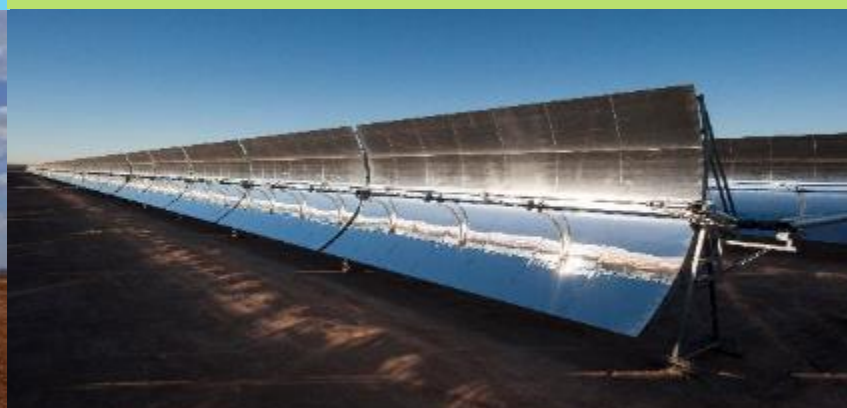
Ashalim Solar CCP (Israel) – 1344 uts
